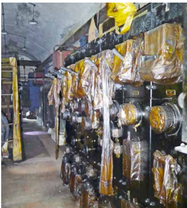
Fire Control South: switchgear in the eastern engine room
